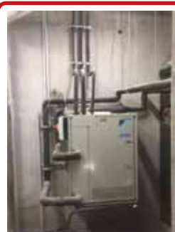
Water cooled condensers
