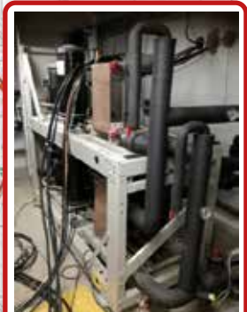
Water cooled chiller for air processing in the AHUs
