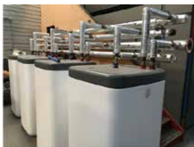
Heat recovery (HR) Plant Melbourne C&P
