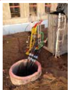
All equipment is using geothermal loop (also the one installed in “The Eye” part)
