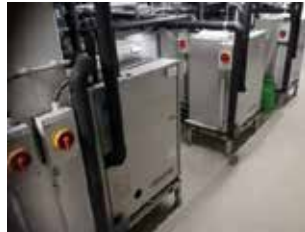
Water cooled condensers for dimatization of all the rooms of “The Brow”
